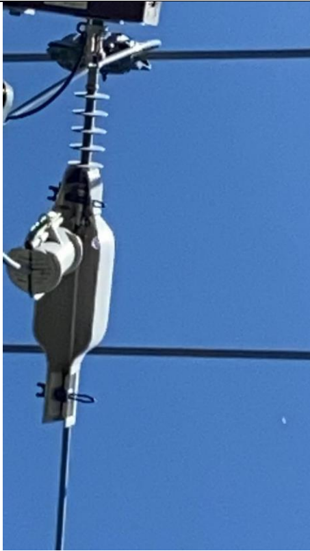
Item7IA2Img1: No anti-rotational clip installed on dead end cover
