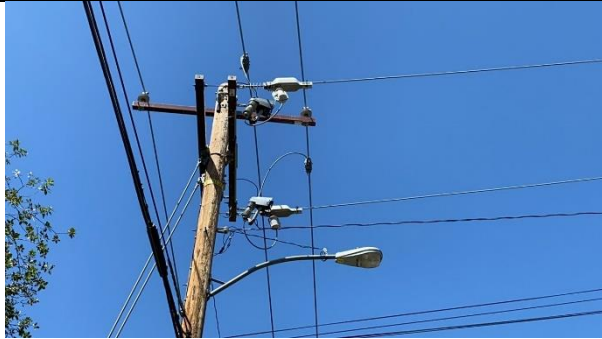
Item7IA1mg1: No vibration dampers
