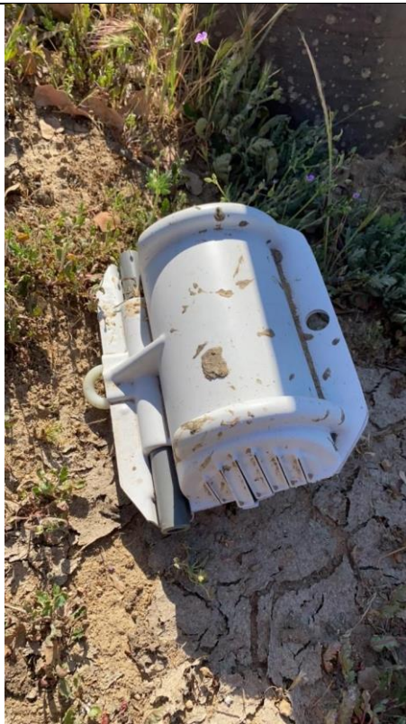
Item3IA1Img1: Wildlife terminator/pothead on ground next to pole
