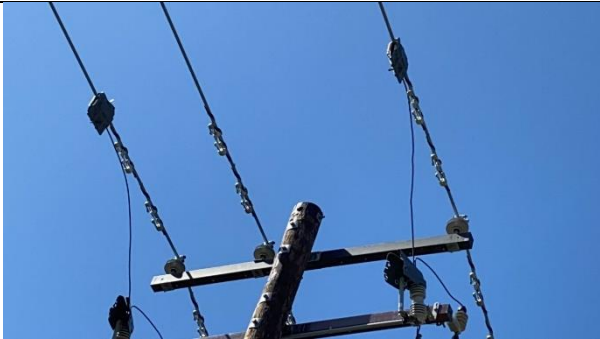
Item5IA1Img1: Observation: Vibration dampeners installed between bolted wedge connector cover and crossarm
