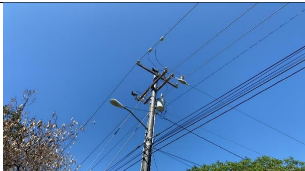
Item6IA1Img1: No vibration dampers
