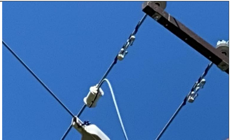
Item4IA1Img2: Observation: Close up showing vibration dampers on upper pole phase level between jumper and crossarms
