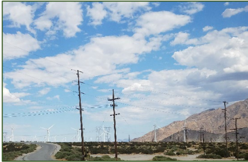
Shown: Shrubs Under Utility Lines, Palm Springs
