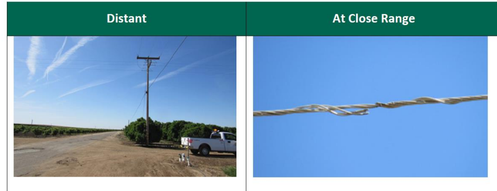
Damaged Primary Conductor on a 12kV Circuit
