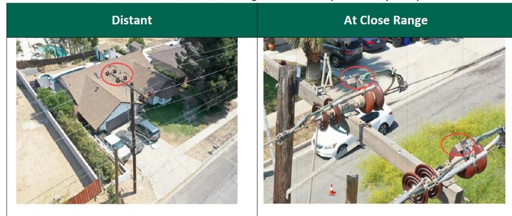
Distribution Switchblade Alignment Issue (Drone Capture)
