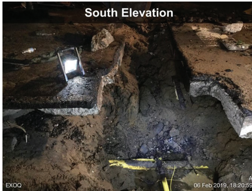
Figure 7: (from Exh 13 ) Damage at branch connection. Courtesy PG&E.
