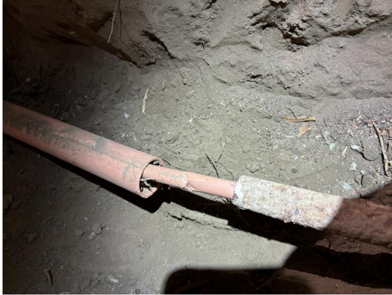
Photo 32: Provided by Southern California Gas Company, showing a close up of damaged 0.5-inch plastic natural gas pipeline. (Exh. 1.)
