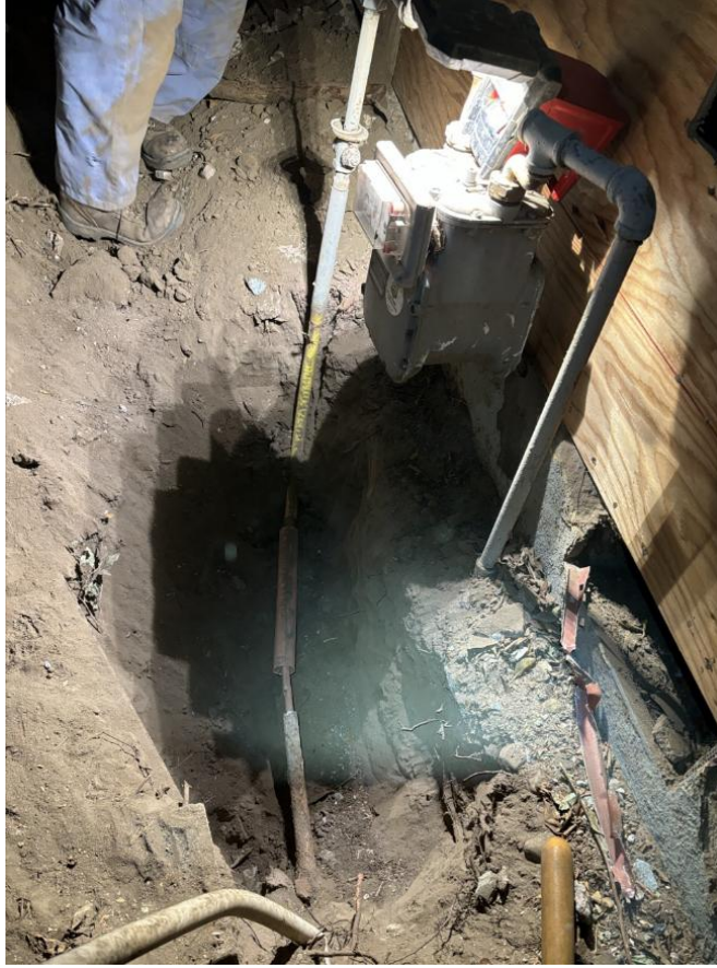
Photo 11: Provided by Southern California Gas Company, showing the damaged natural gas pipeline. (Exh. 1.)
