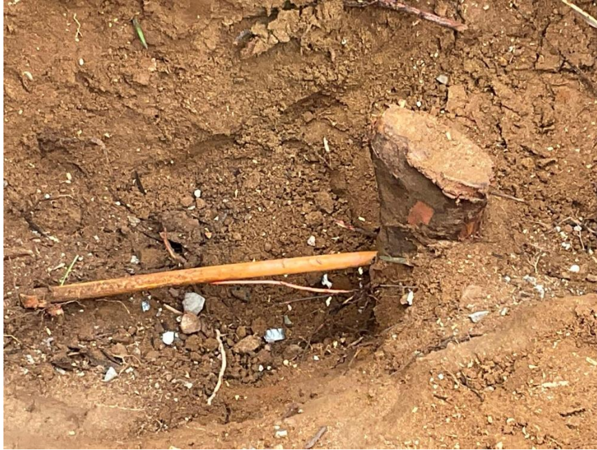
Photo 2: Provided by San Diego Gas and Electric, depicts the damaged 0.5-inch plastic natural gas pipeline.
