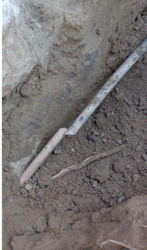
Photo 1: shows the completely severed 1/2" plastic natural gas facility, in the ground, provided by SoCalGas. (Exh. 1.)
