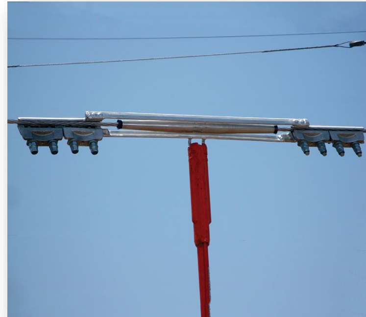
Transmission shunt installation
