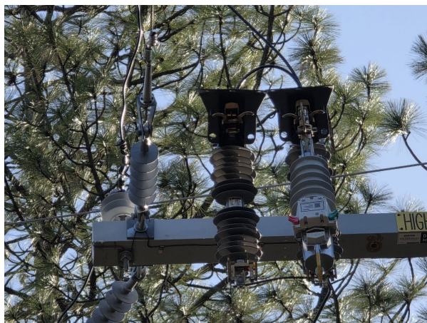
Figure 7: Example Non-Exempt Expulsion Fuse Removal Field Images
