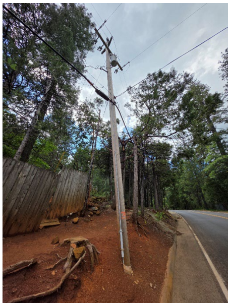
Figure 8: Communication Guy Wire Field Images
