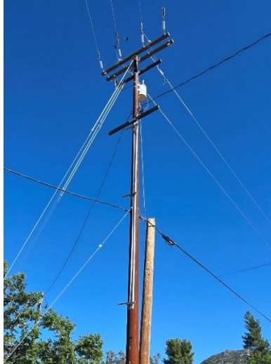
P43751 C448 – Cross-Arm, Brackets, and Conduit Installed without SCADA Equipment
