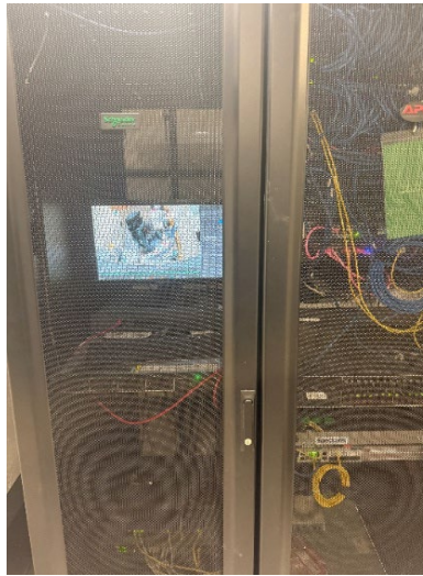
Server Room Equipment
