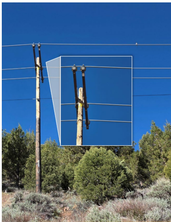
Structure # Circuit Number 1026BV Baldwin 34kV
