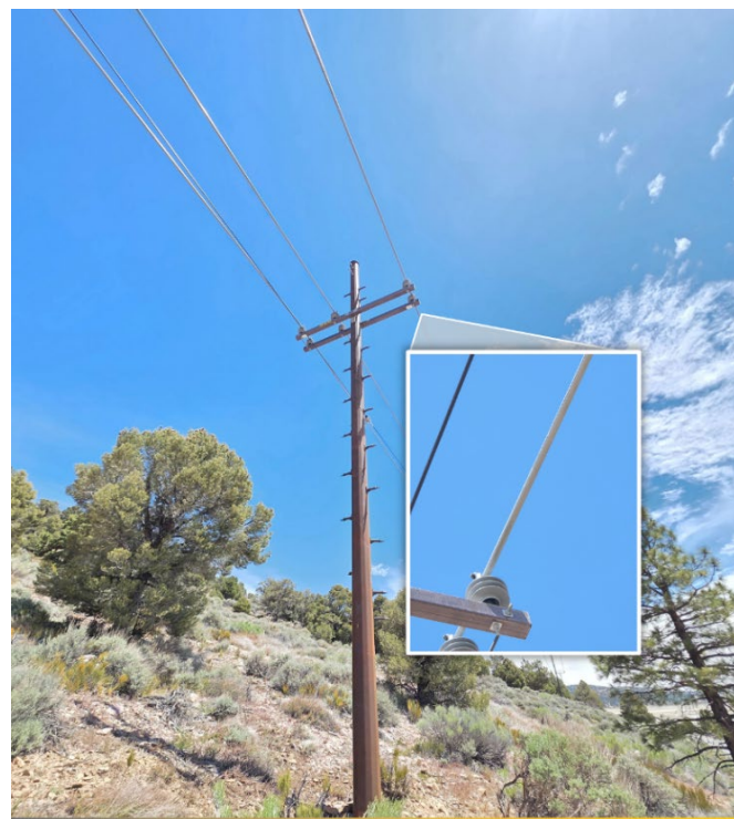
Structure # Circuit Number 15542BV Baldwin 34kV
