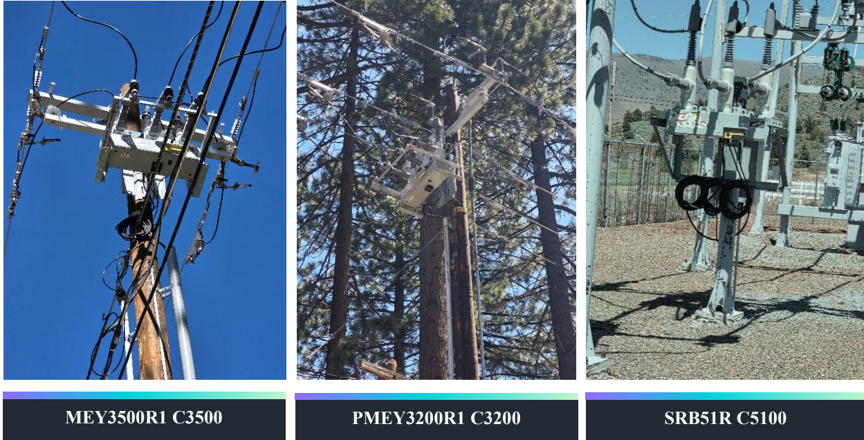
Figure 6: Example of System Automation Equipment Field Images
