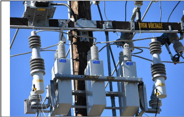
Asset Image 1: Missing capacitor bushing cover
