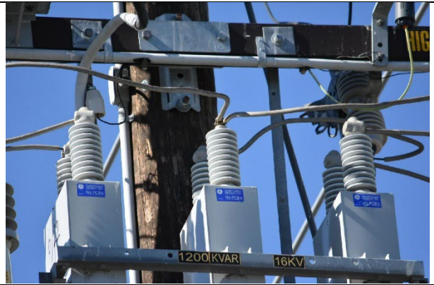
Asset Image 2: Missing capacitor bushing cover
