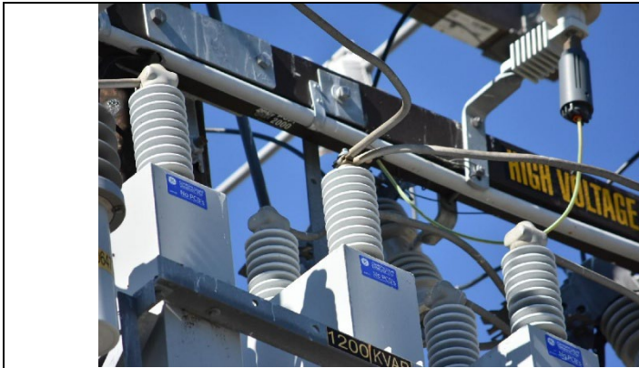
Asset Image 3: Missing capacitor bushing cover
