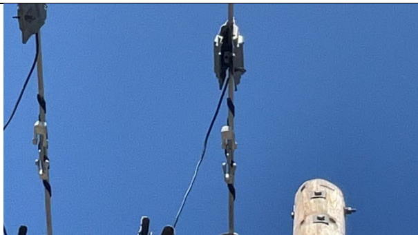
Asset Image 2: View of unsecured tap cover
