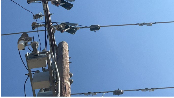
Asset Image 3: View of unsecured tap cover
