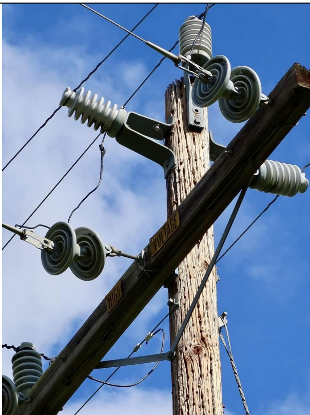
IA1Img3: WP damage 3.
