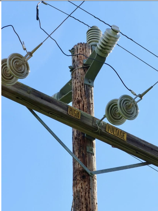
IA1Img1: WP damage 1.
