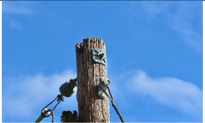
IA1Img3: Span/down guy anchor on decaying pole.
