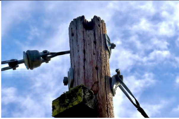
IA1Img2: Large piece of pole missing near critical strain point within 6" from top.
