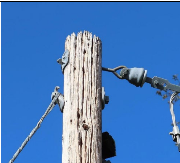
IA11mg1: Evidence of pole decay.
