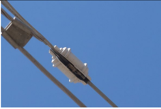
Asset Image 3: View showing unsecured tap cover and exposed bare wire
