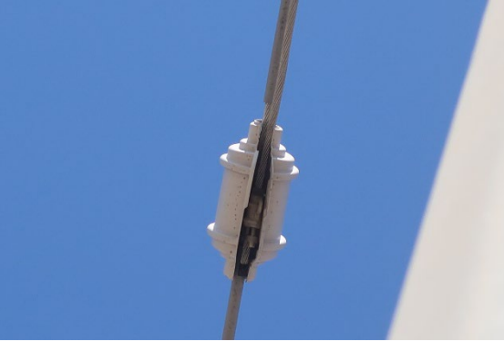
Asset Image 5: View showing unsecured tap cover and exposed bare wire
