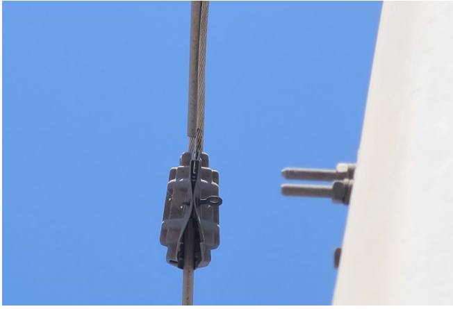
Asset Image 3: View showing exposed bare wire next to avian protection cover
