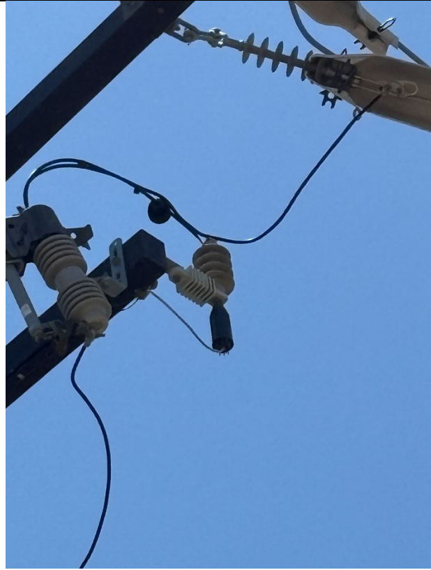
Asset Image 2: View showing dislodged lightning arrester cover
