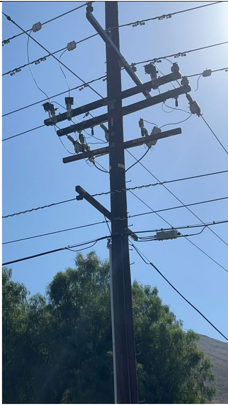
Asset Image 1: View showing dislodged lightning arrester cover
