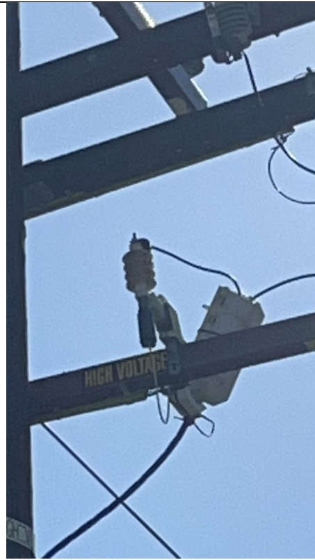
Asset Image 2: View showing dislodged lightning arrester cover
