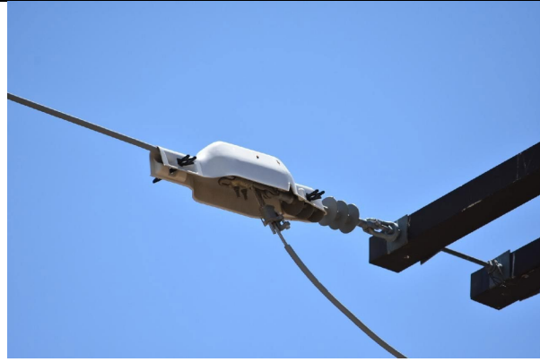
Asset Image 3: Missing connection cover
