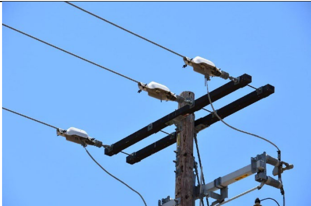
Asset Image 1: Missing connection covers
