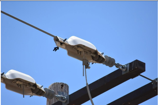
Asset Image 2: Missing connection cover
