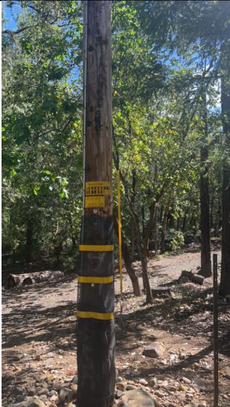
Photo 2: Photo of pole ID 06246011.0181505.
