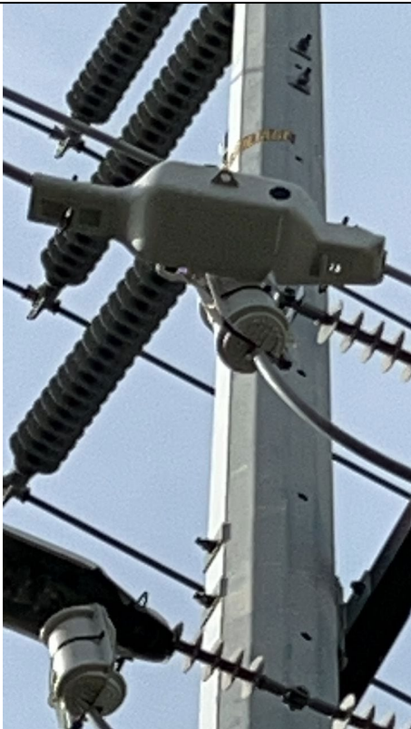
IA1Img3: Dislodged wildlife cover (close-up view)
