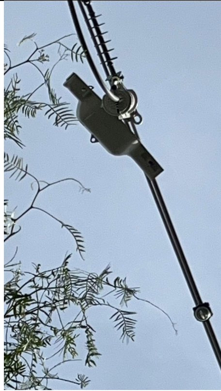
IA1Img2: Dislodged wildlife cover (close-up view)
