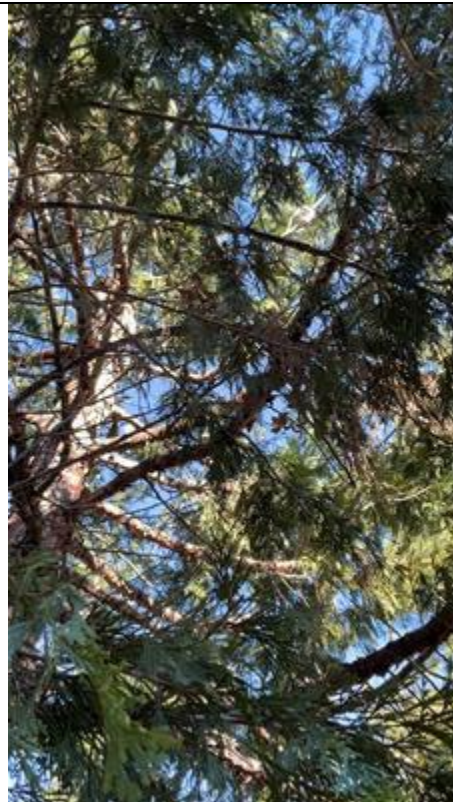
IA1Img4: Vegetation in contact with the guy wire above the insulator
