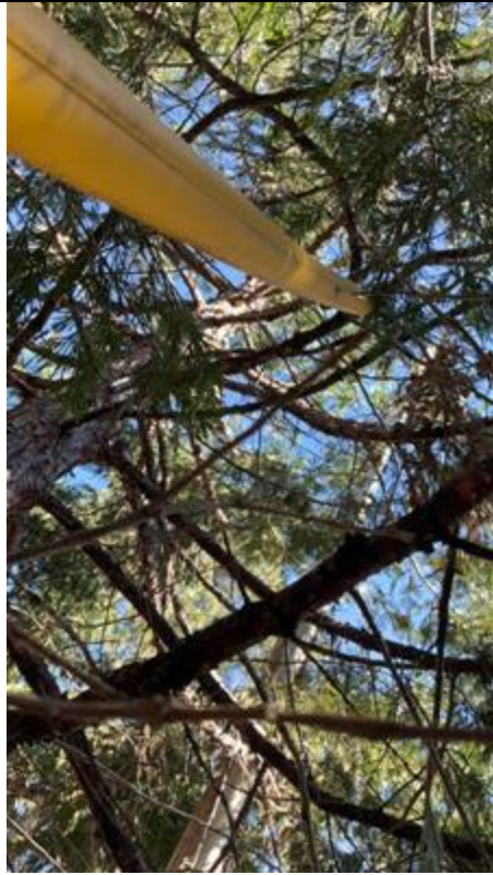
IA1Img6: Vegetation in contact with the pole and guy wire
