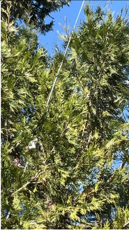
IA1Img5: Vegetation in contact with the guy wire above the insulator
