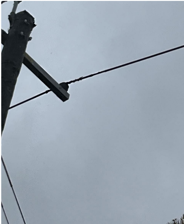
IA1Img3: Another phase showing tape applied over the conductor on the southeast side of the pole 121528551
