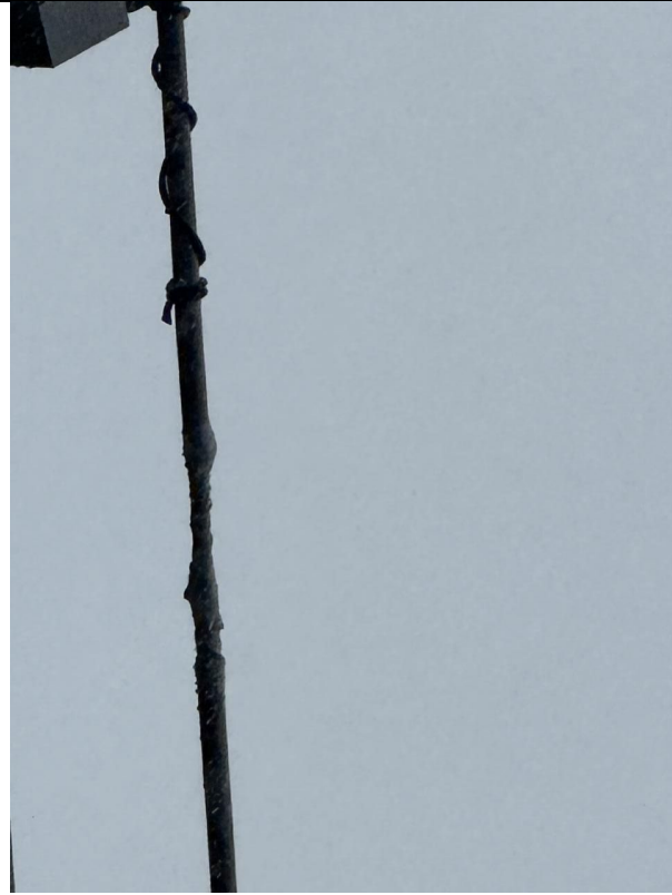
IA1Img2: Close up view of one phase showing tape applied over the conductor on the southeast side of the pole 121528551
