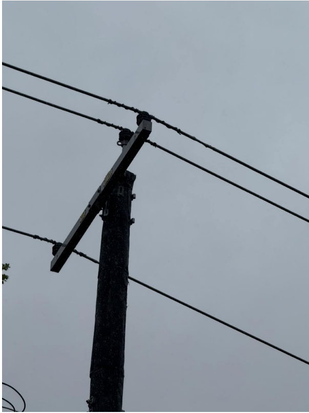
IA1Img1: Overall view showing tape applied over the conductor on the southeast side of the pole 121528551.
