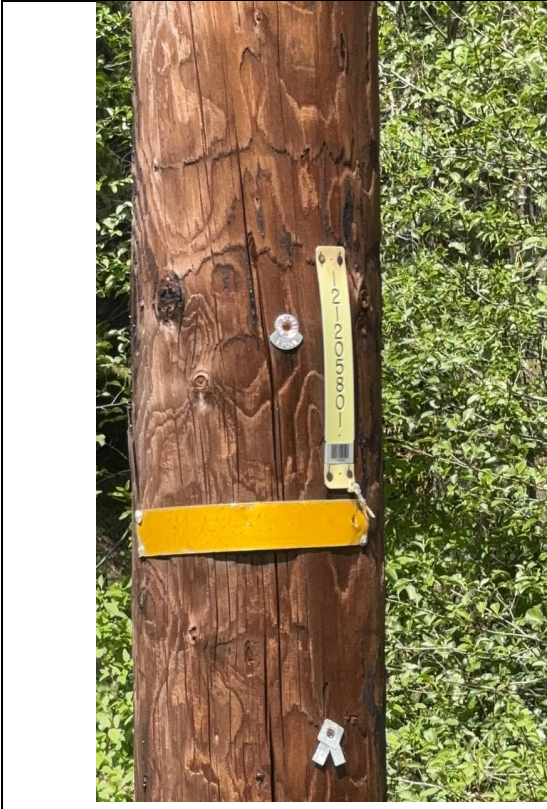
Photo 1: Photo of pole ID 121205801.
