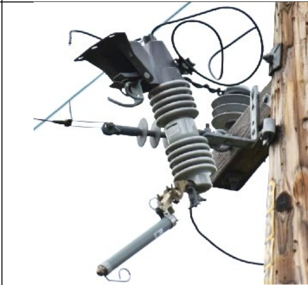
IA1mg2: Exempt fuse is disconnected and unplugged (close view).
