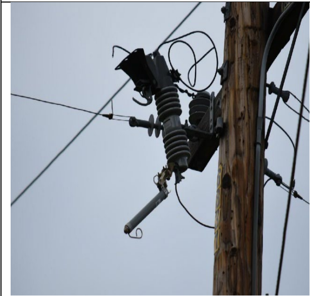
IA1mg1: Exempt fuse is disconnected and unplugged.
