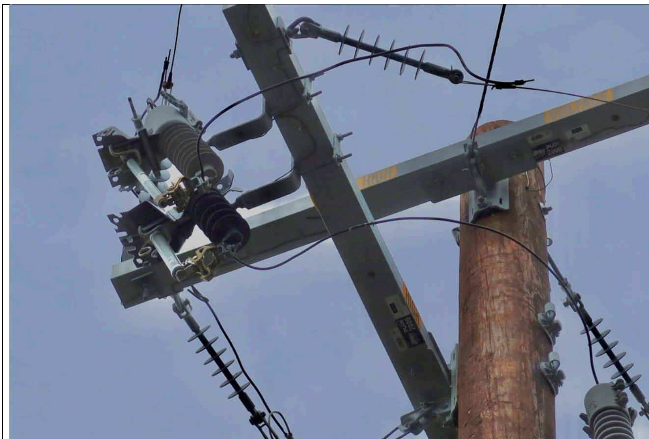
IA1Img3: Elf Fuse going to transformer bushing, non-exempt fuse going to line.
