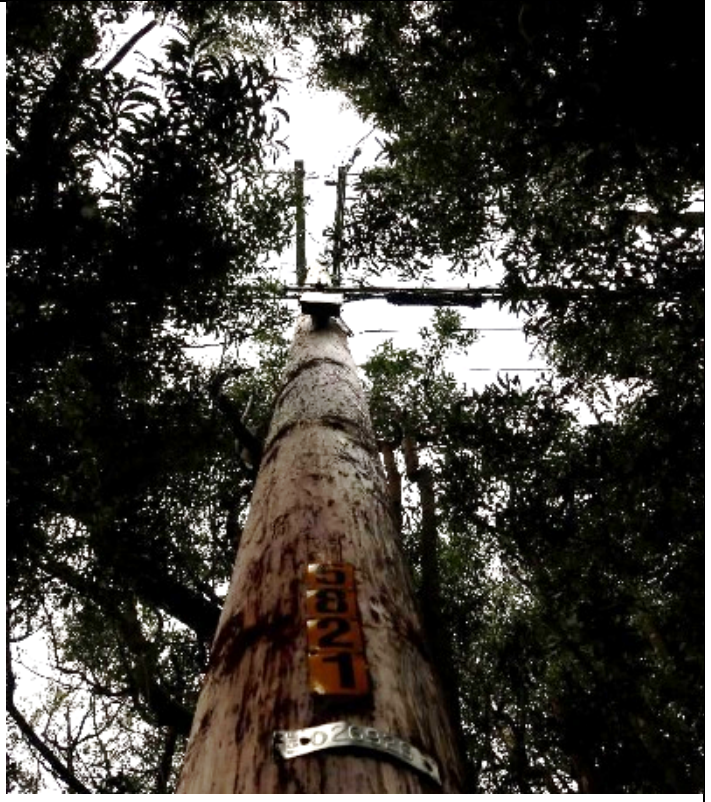
IA1Img2: Solid Blade Disconnects and lack of reclosers, sectionalizers, or voltage regulators.
