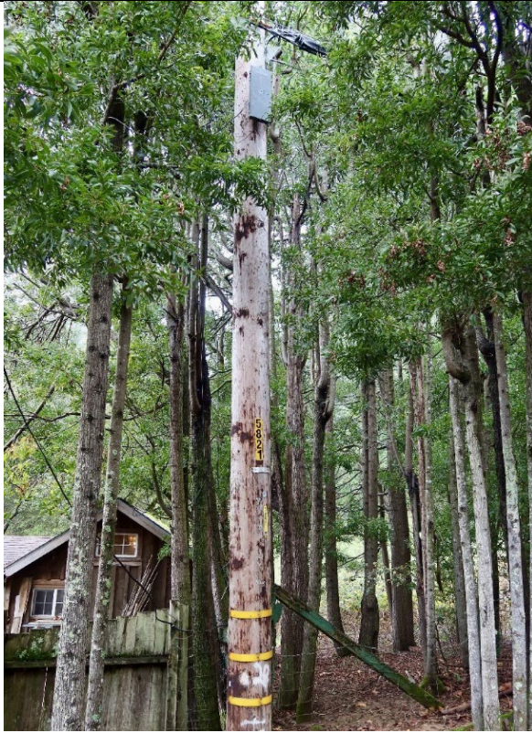
IA1Img1: Solid Blade Disconnects and lack of reclosers, sectionalizers, or voltage regulators.
