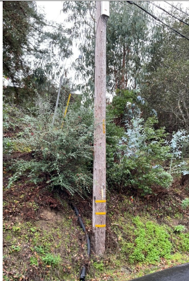
IA1Img1: Pole with vegetation within 10 feet of the base.
