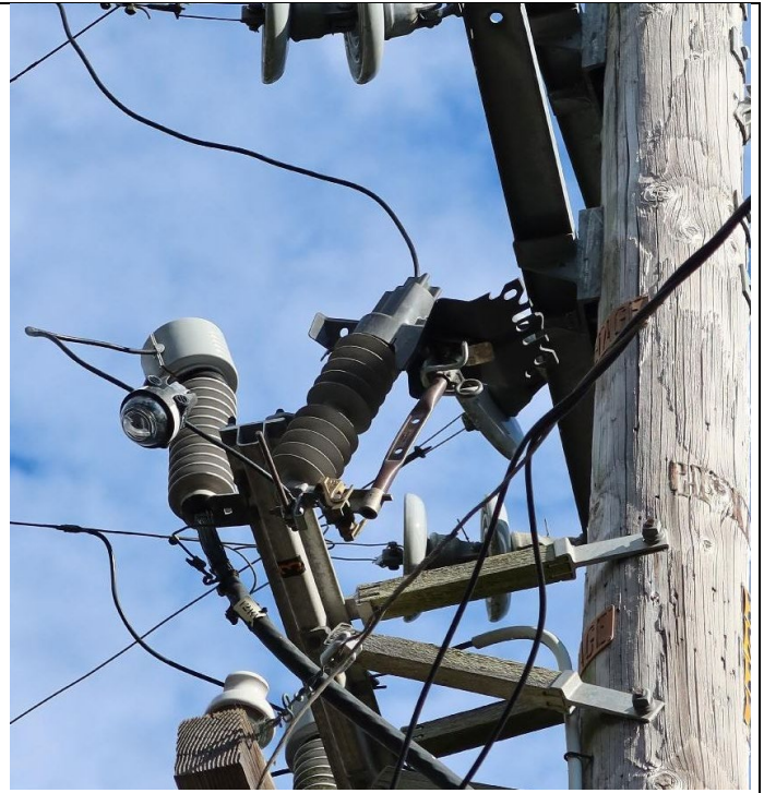
IA1Img2: Solid blade disconnects (Close View).
