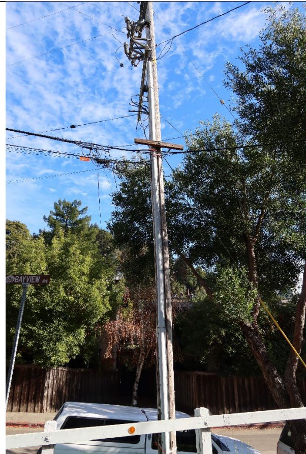
IA1Img4: Solid Blade Disconnects and lack of reclosers, sectionalizers, or voltage regulators.
