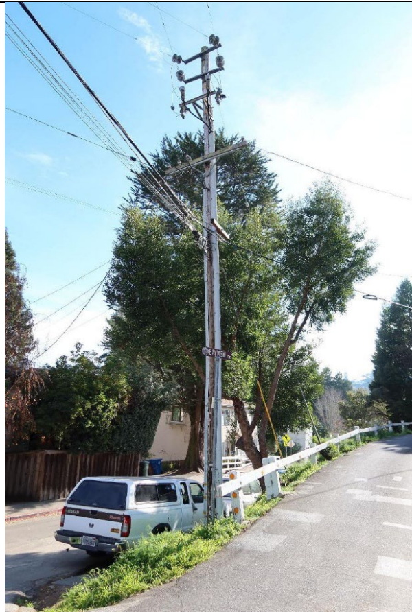
IA1Img3: Vegetation within 10 feet of the base of the pole.
