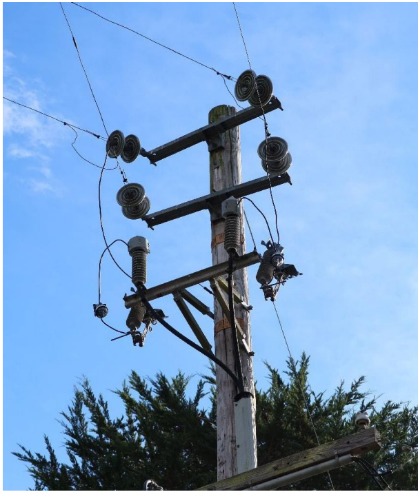
IA1Img1: Solid blade disconnects.
