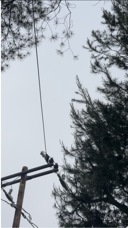
Photo 5: Additional photo of the pine tree within the four-foot minimum clearance distance from the primary conductor. Photo taken from under the primary conductors.
