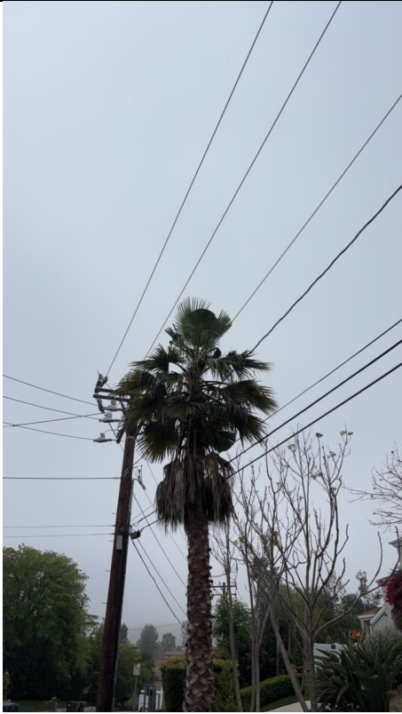
Photo 3: Photo of the Mexican palm tree growing under the conductors and within the four-foot minimum clearance distance. Photo taken south of the tree looking north.
