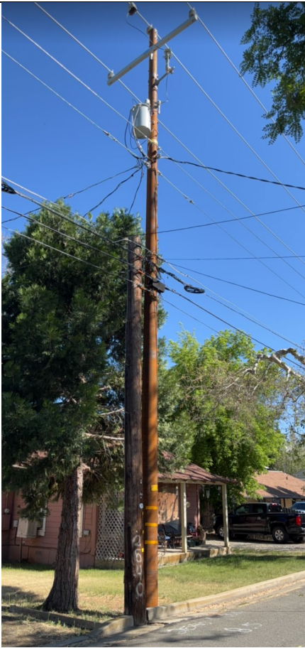
Data Inaccuracy Img10-1: No system automation installed
