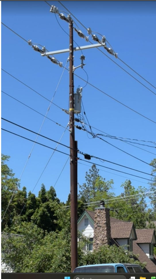
Data Inaccuracy Img6-1: No system automation installed
