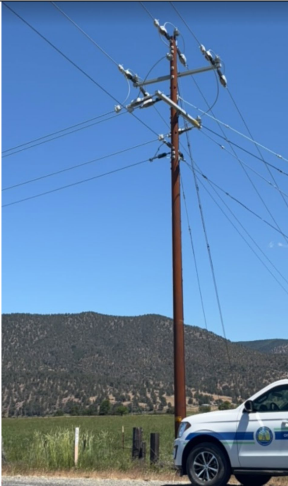
Data Inaccuracy Img2-1: No system automation installed
