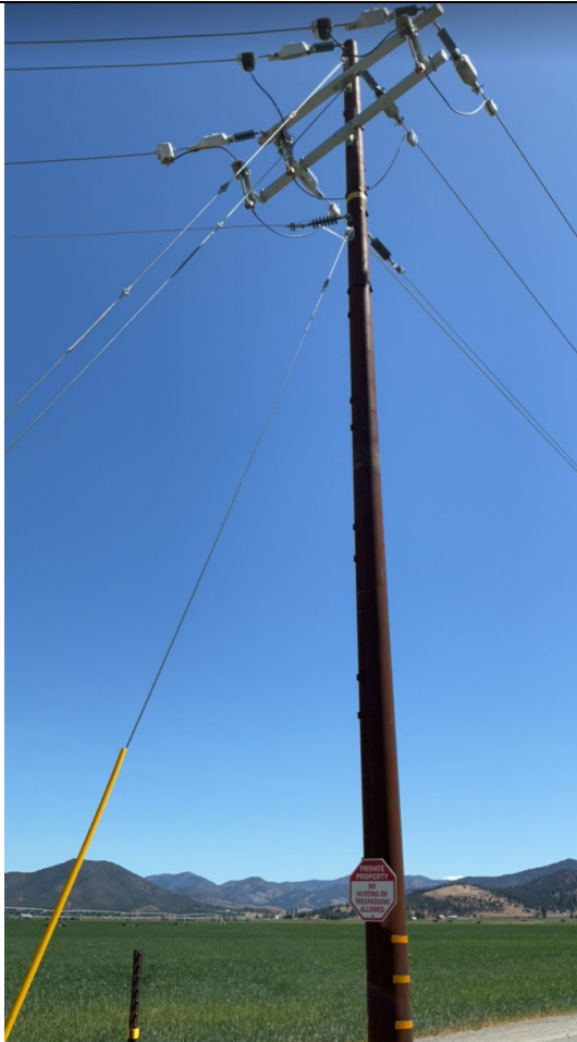
Data Inaccuracy Img12-1: Two expulsion fuse replacement initiatives have been submitted at this location for the same quarter Q4.
