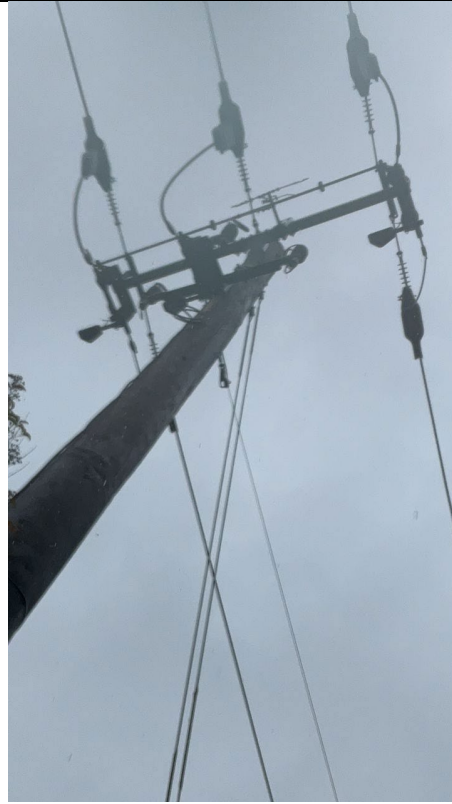
IA1Img2: Close up view of pole 121901742 showing a bare conductor on the west side of the middle phase
