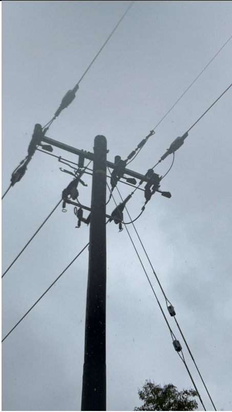
IA1Img1: Close up view of pole 121901742 showing a bare conductor on the west side of the middle phase
