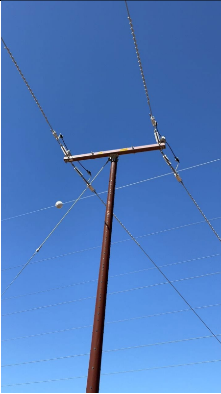
Asset Image 1: Lighting arresters not present
