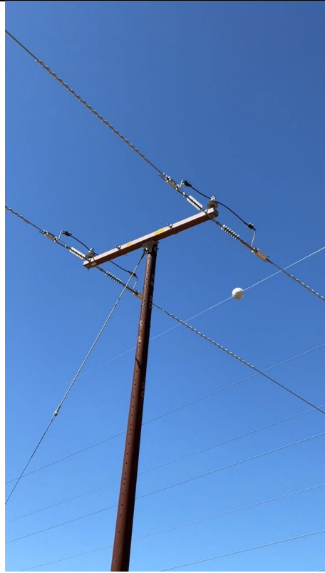
Asset Image 2: Lighting arresters not present
